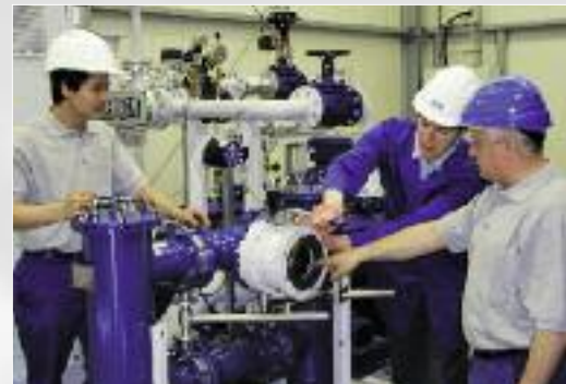
Commissioning and training by Lechler staff
