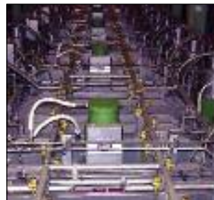
MasterCooler SMART® in slab plant
