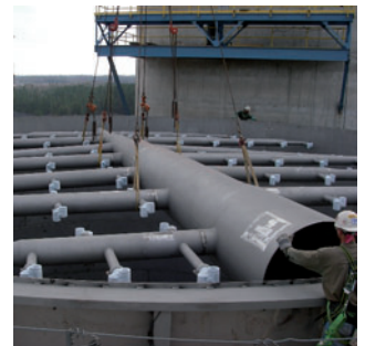
Customized configuration according state-of-art-technologies
