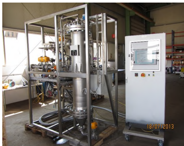
Pilotanlage inkl. Schaltschrank / Pilot plant with control board
