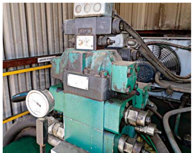
Figure 6. Inspecting hydraulic systems for leaks frequently is an important aspect of system maintenance, but leak reduction can also cut down on contamination ingress.
